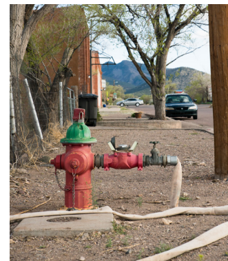
Detail of fire hydrant.
