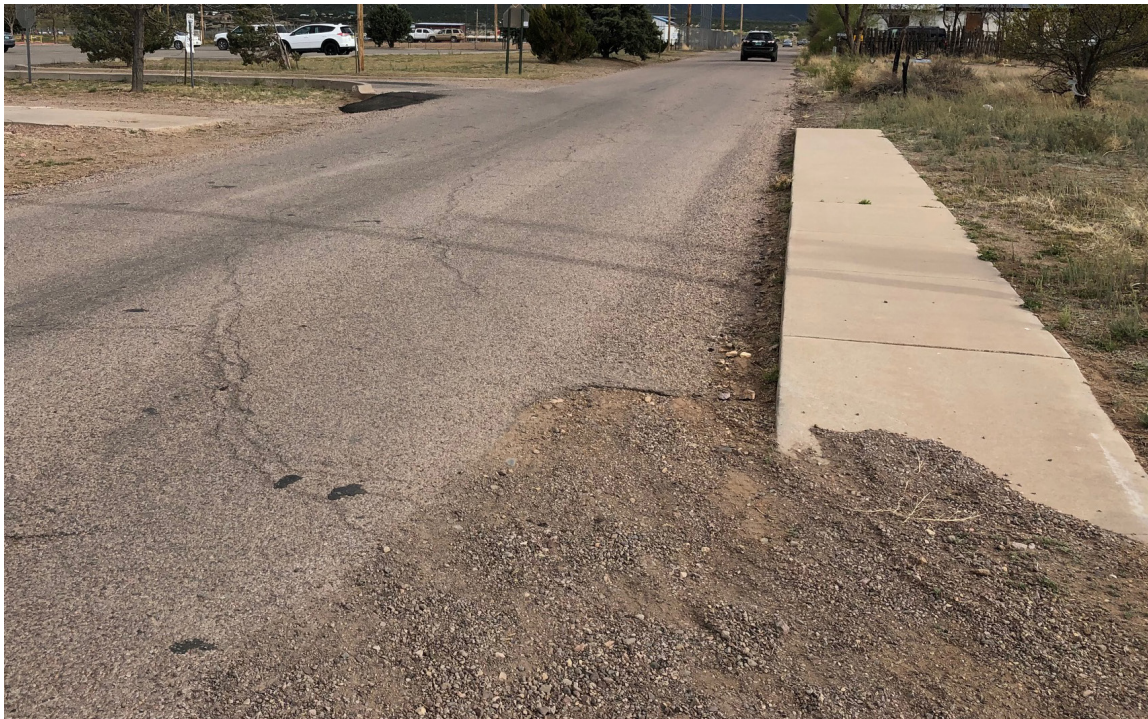
Gravel trip hazard along Duggins Drive.
