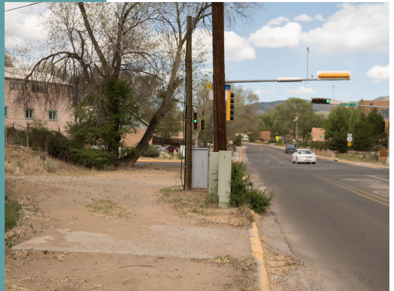
Shoulder/partial sidewalk on Ranchitos Road is obstructed by power lines and electrical boxes.
