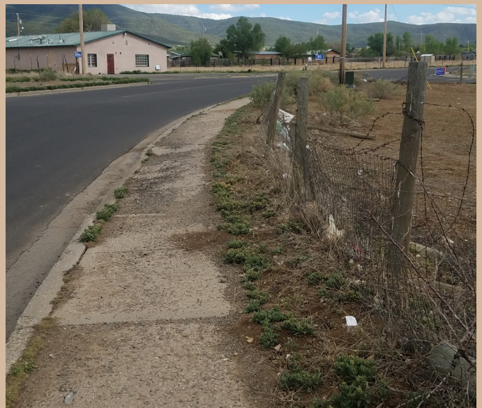
This sidewalk near Los Pandos and GUSDORF Roads is poorly maintained.
